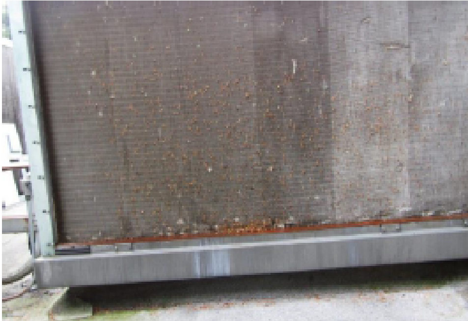
Police Station: ACU-1 past its 15-year useful service life.
