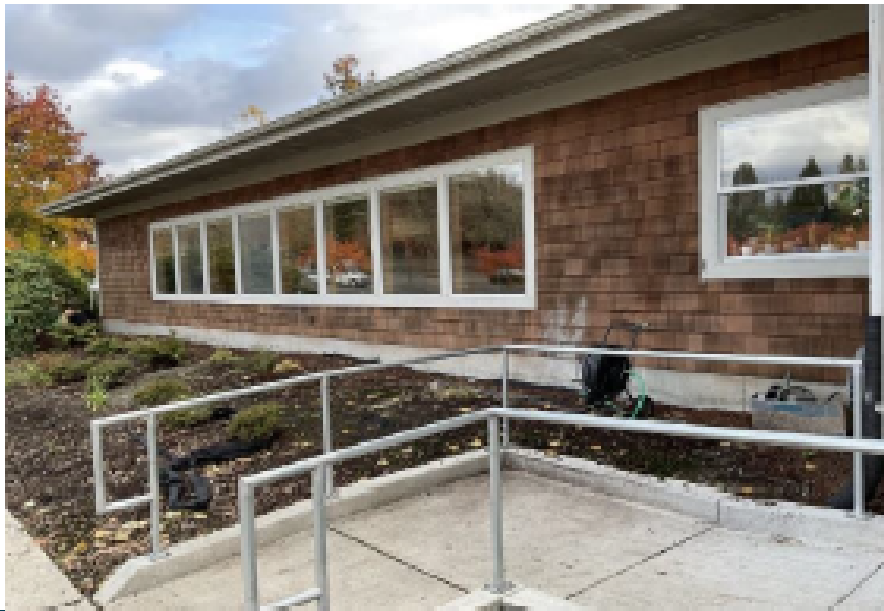
Mickey Corso Community Clubhouse: Exterior siding is past its useful service life, and has areas of significant wear and damage.
