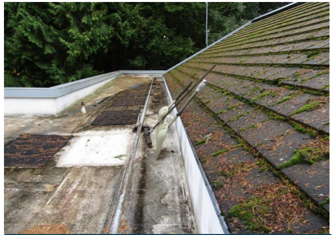
Library: Moss growth on concrete shingles.
