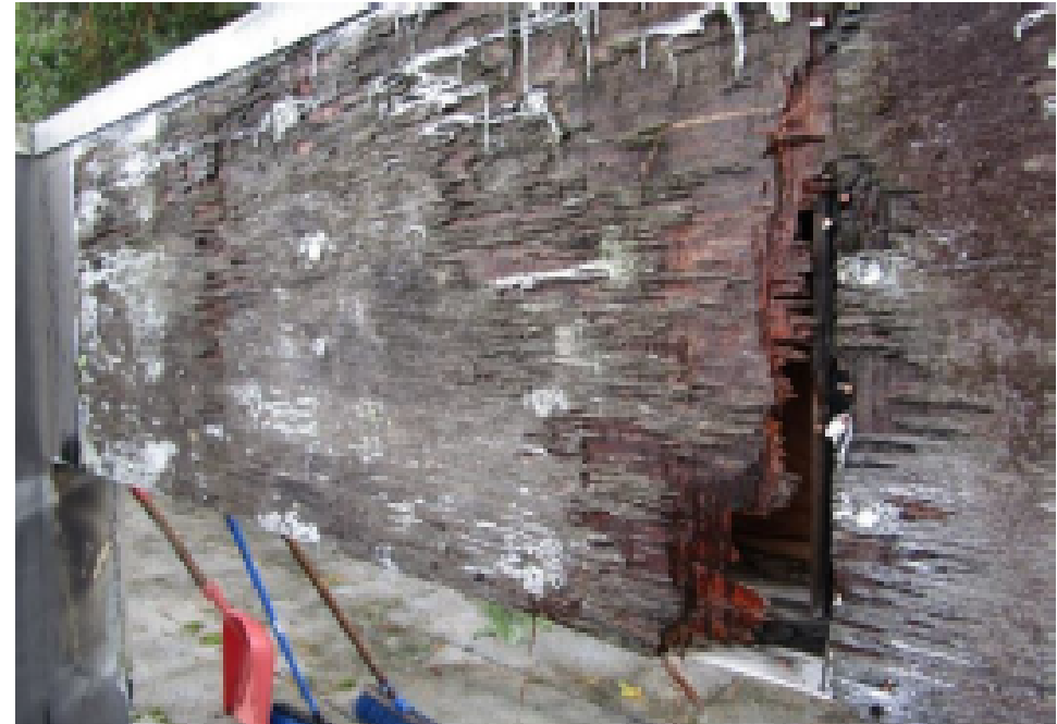
Police Station: Wood partition surrounding the rooftop unit is damaged.
