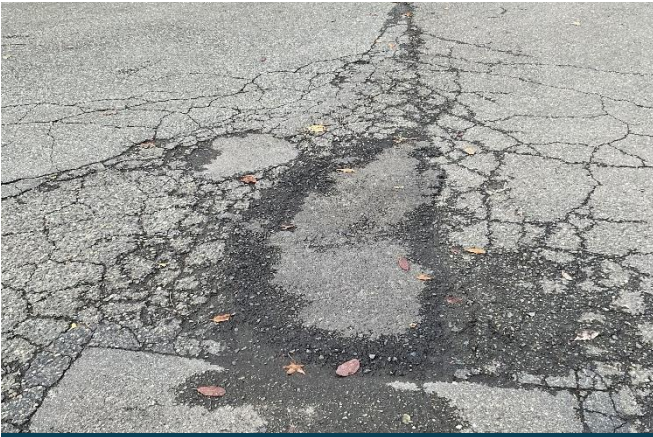
Mickey Corso Community Clubhouse: Parking lot has alligator cracking, damaged curbs and needs repainting.
