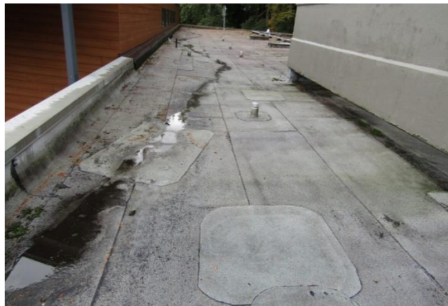
Police Station: Roofing damaged and worn with multiple patches.
