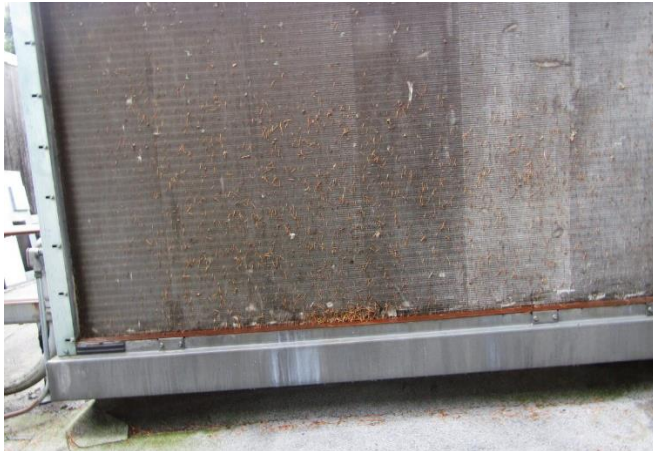
Police Station: ACU-1 past its 15-year useful service life.
