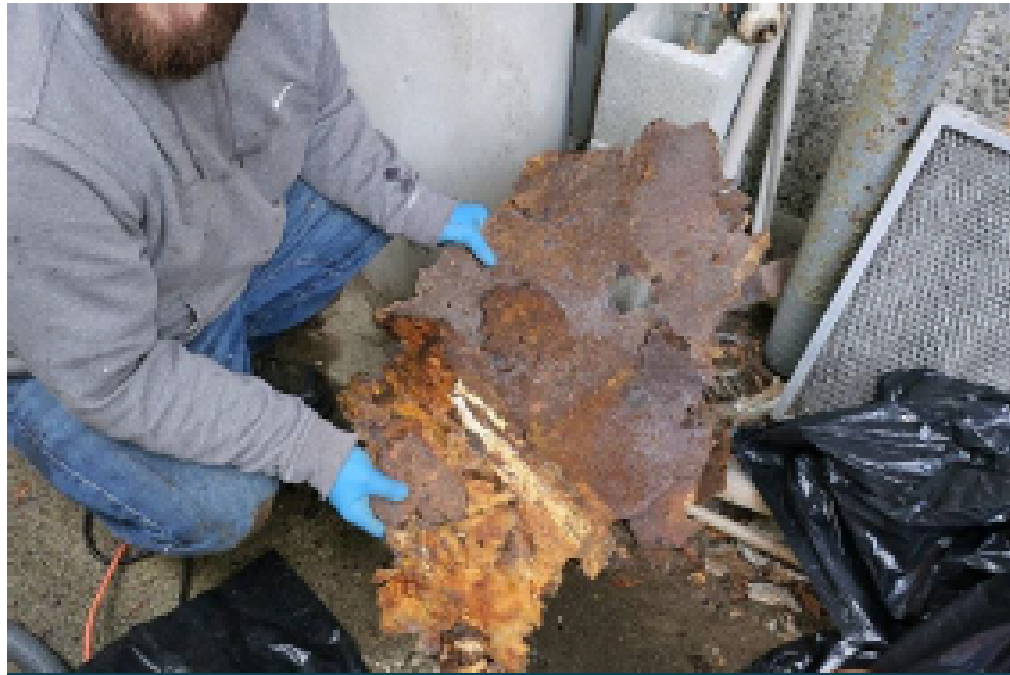
Recreation Pavilion: Rusty metal removed from HRU-1 interior.
