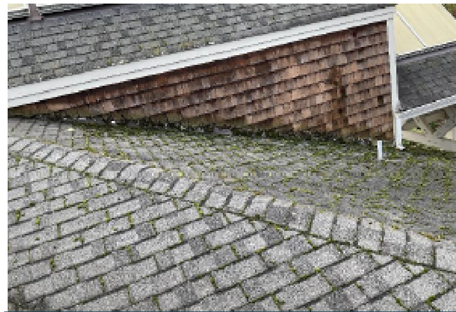
Mickey Corso Community Clubhouse: Roof has moss growth and shingles have exceeded expected useful life.
