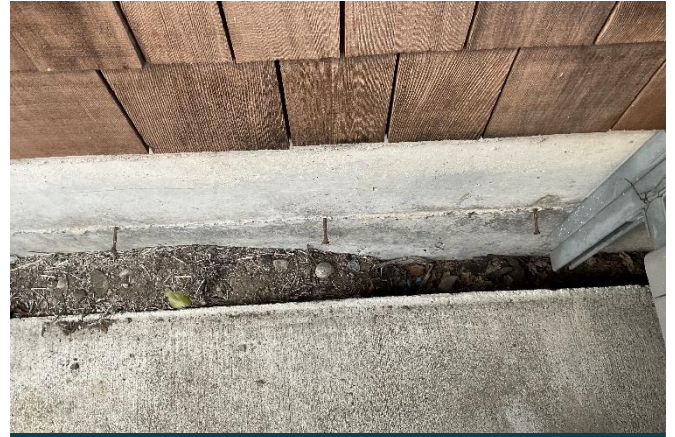
Mickey Corso Community Clubhouse: The concrete patio surrounding the building is separating from the building foundation.
