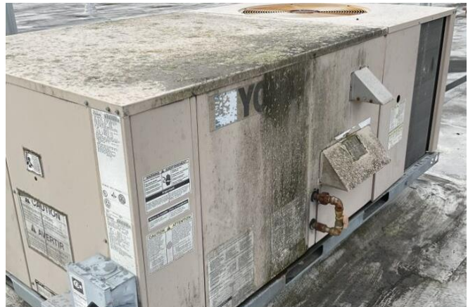
Operations Facility: Rooftop package unit past its industry expected life.
