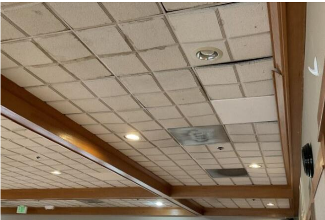
Mickey Corso Community Clubhouse: Lay in ceiling tiles show significant wear and some damage.
