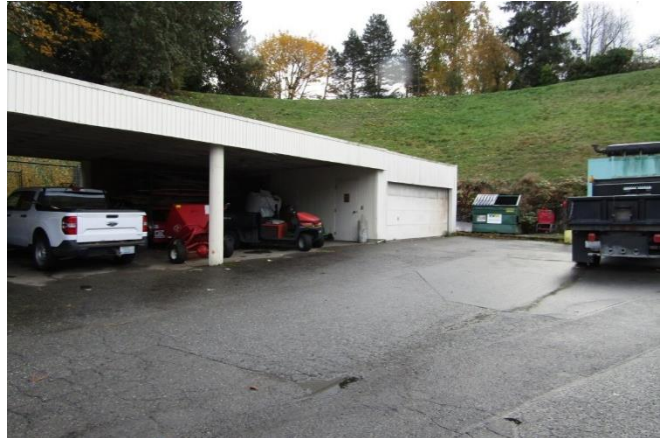
Operations Facility: Carports are in poor condition.
