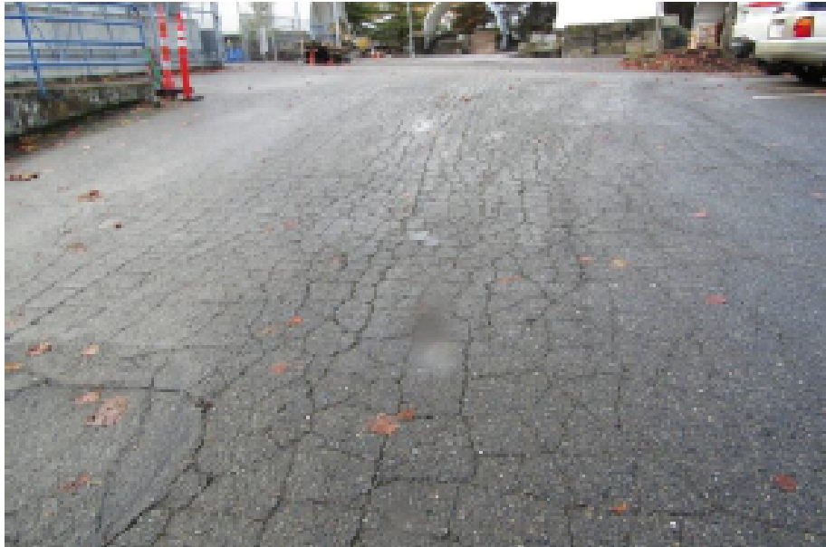
Operations Facility: Parking lot has alligator cracking, damaged curbs and needs repainting.
