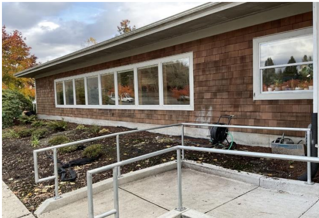
Mickey Corso Community Clubhouse: Exterior siding is past its useful service life, and has areas of significant wear and damage.
