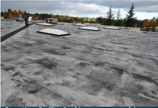
Operations Facility: Roof has many areas of damage and wear, prior patching, and leaks.
