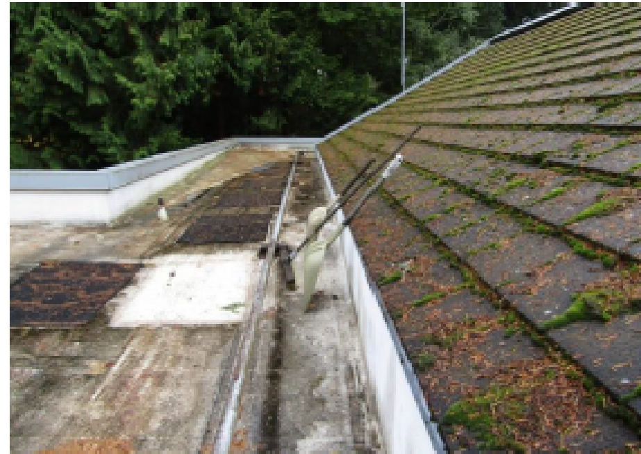
Library: Moss growth on concrete shingles.
