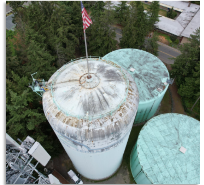
Water Storage Tanks
