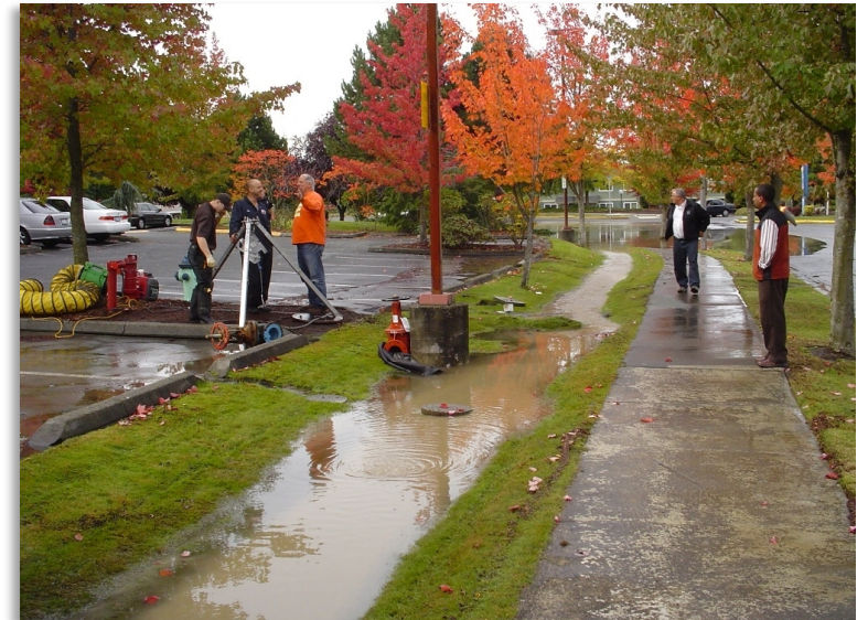
Post-Flooding Clean Up
