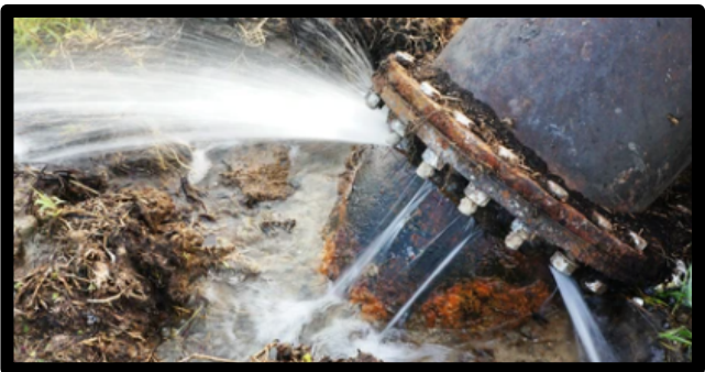
Likely End of Useful Life for MLT Pipes?
